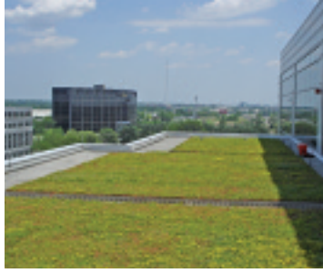
Green roof embedded at Calamos Investments office in Napierville, Illinois (Photo courtesy of Green Roofs for Healthy Cities)
